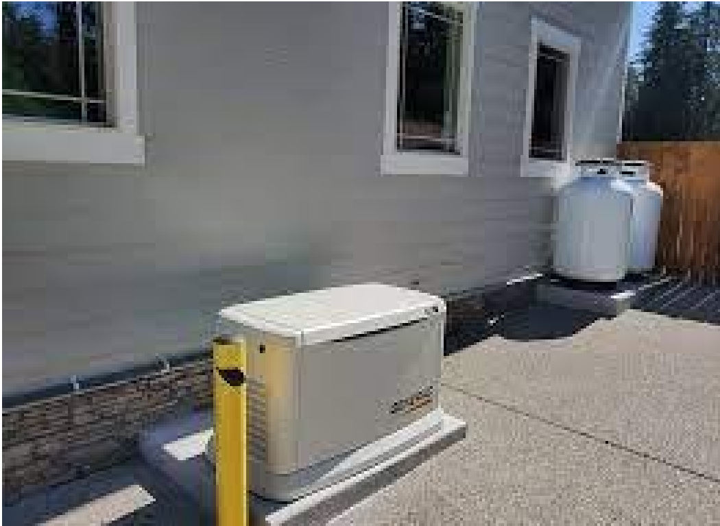
FIGURE 5 – EXAMPLE OF CONCRETE PADS WITH FUTURE PROPANE TANKS AND GENERATOR
